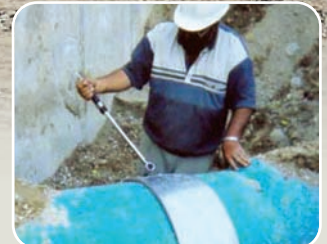
▲ UK: buried water supply pipes
