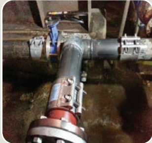
▲ Netherland desalination treatment facilities
