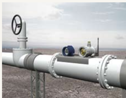
Landfill Gas Flow Control
